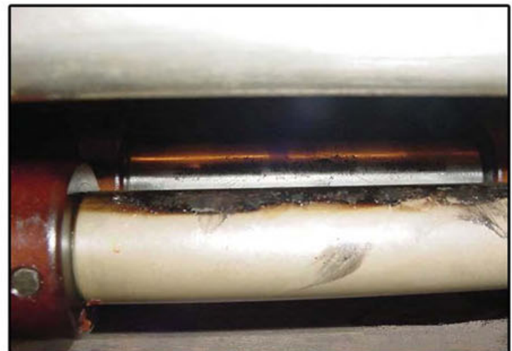
Figure 4. - Burn mark on in-tank LTC component
