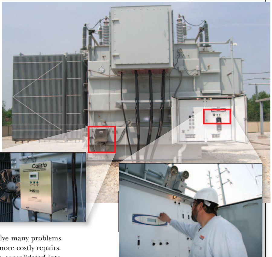
Monitoring is installed on more than 130 transformers over 40 MVA. The left insert shows the dissolved gas-in-oil and moisture-in-oil sensor. The right insert shows an engineer using the Dynamic Ratings system control panel.
